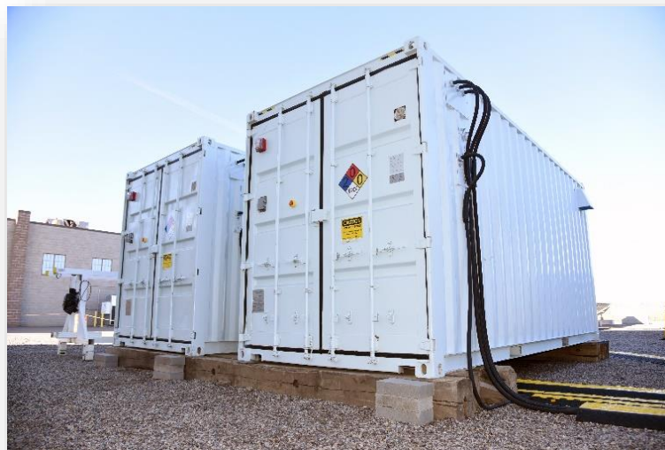
Figure 6: Flow Battery at INL's microgrid test bed; Photo by Idaho National Laboratory; CC BY 2.0.
