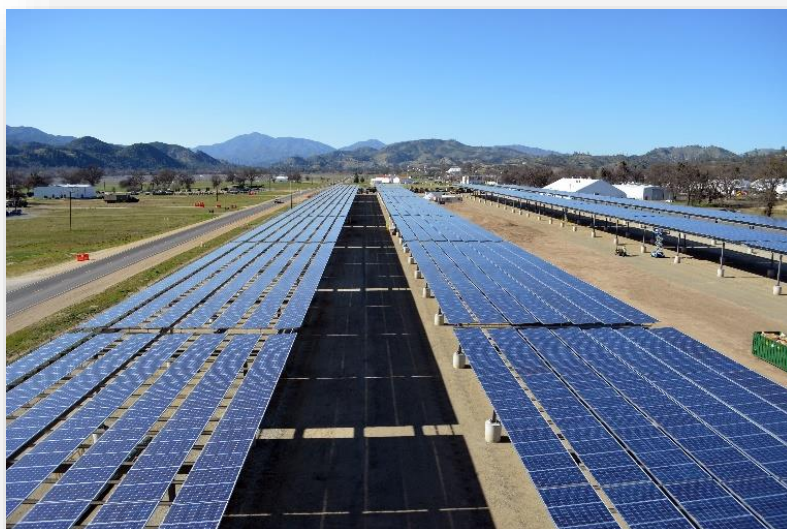
Figure 5: Solar Project at Fort Hunter Liggett; March 2013; U.S. Army Corps of Engineers; Photo by John Prettyman
