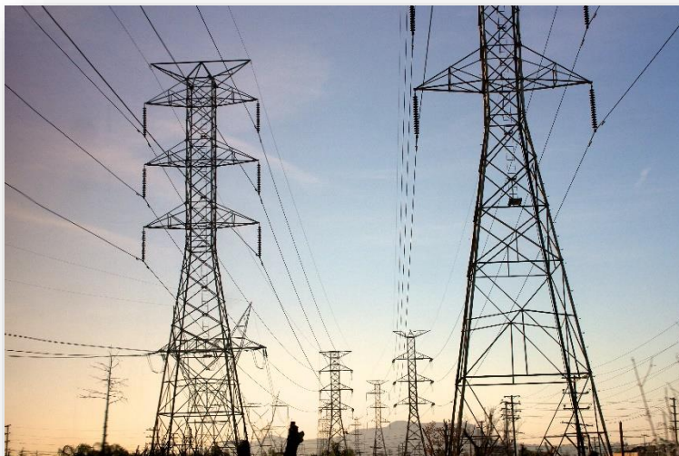
Power Transmission Lines, Photo by Oran Viriyincy, CC By SA 2.0
