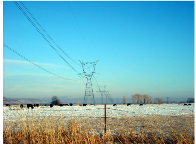
High voltage transmission lines in Duchesne County, Utah. Photocredit: Wikicommons / Staplegunther
