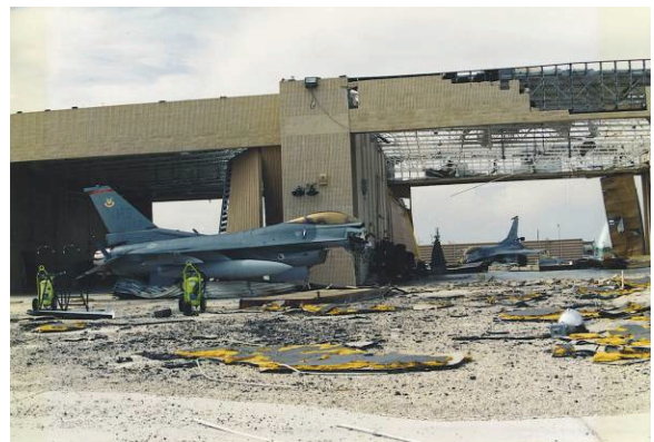
Damage to Homestead Air Force Base after Hurricane Andrew
